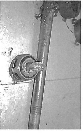
Pump shaft back spinning damage.
